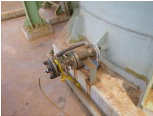
Improper – Remove completely do not left behind the cut portion of the caution tape.
