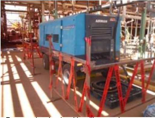
Proper – barricade with railings and provided with access way outside barricaded area.
