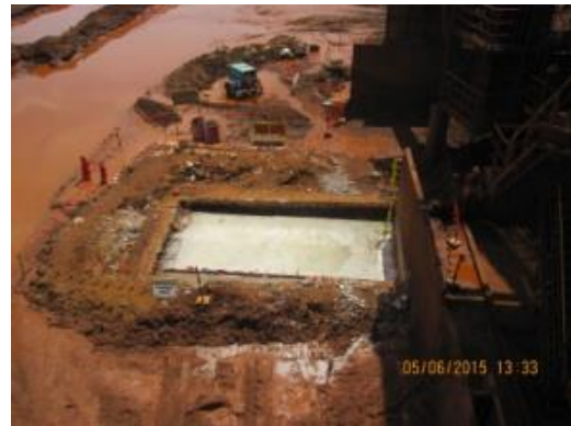
Proper- provided with post, indication tag and access way on excavation area.
