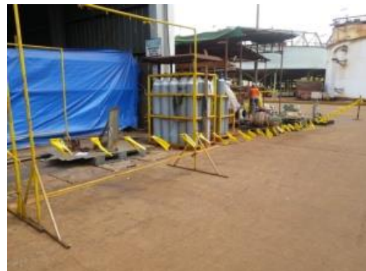
Improper – Low and sagging anybody may overstep and enter the barricaded area. Must install additional post and adjust tension.
