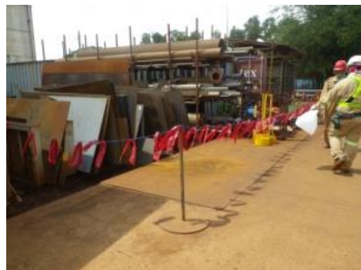
Improper – Should be caution tape not danger tape for storage materials.
