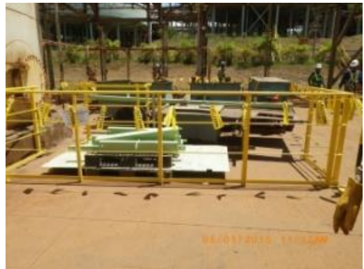
Proper- Full barricade with post and indication tag on temporary storage area.
