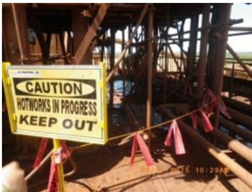
Improper – No access way for other personnel.
