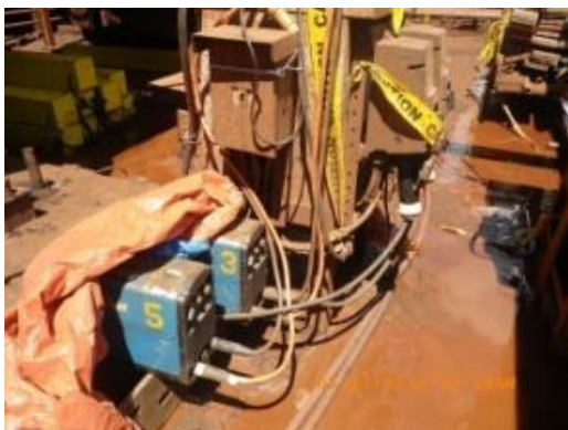
Improper – Not installed on a barricade post.
