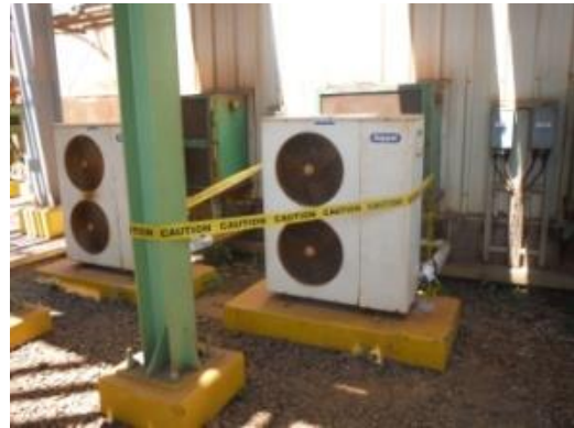
Improper – Not installed on a barricade post.
