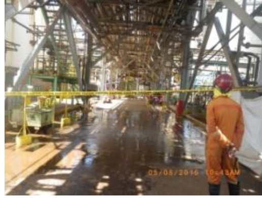
Improper – On going flashing activity barricaded with caution tape must be replaced with danger tape.
