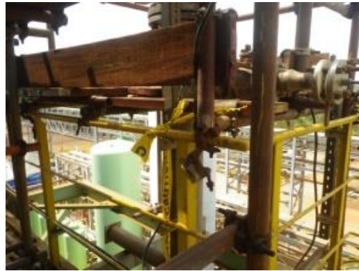
Improper – After activity remove completely do not left behind the cut portion of the tied tape.
