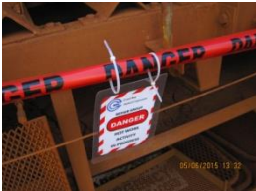
Proper- on going activity with indication tag.
