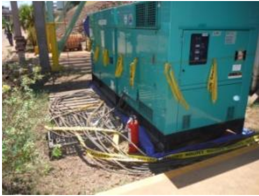
Improper – Not installed on a barricade post.
