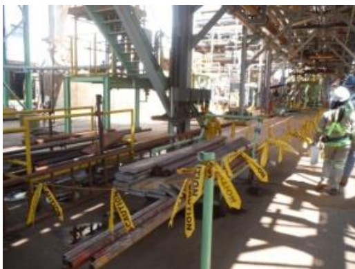
Caution barricade with post, indication tag and access way.
